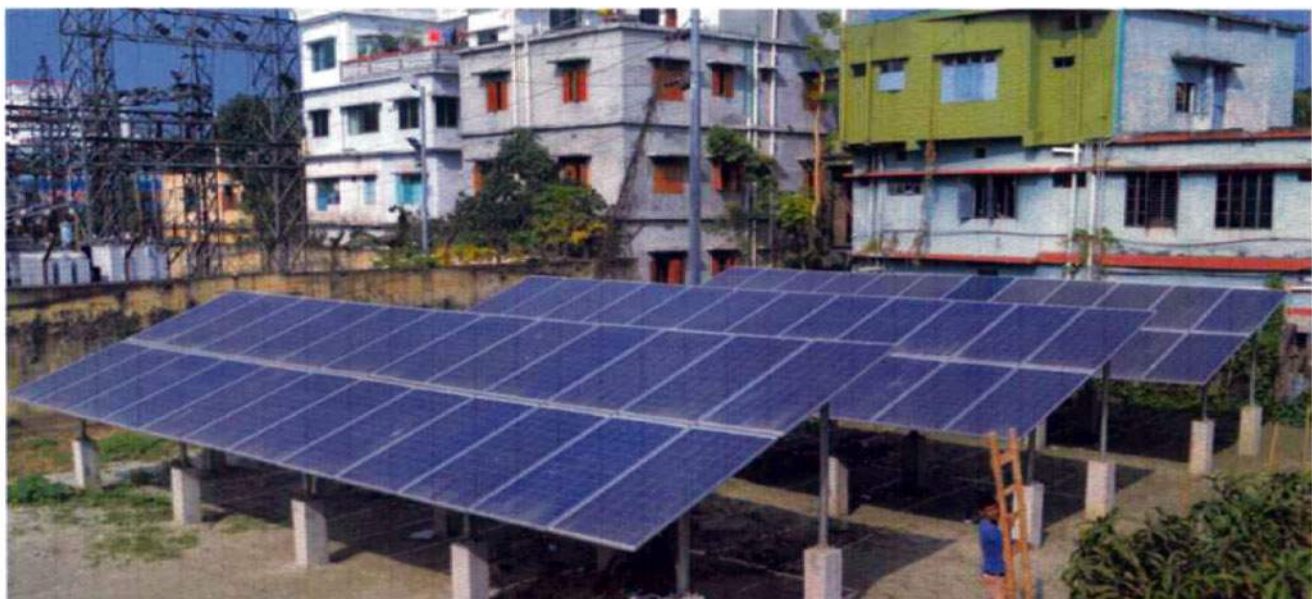
21 kWp Easybike Solar Charging Station, Jashore
