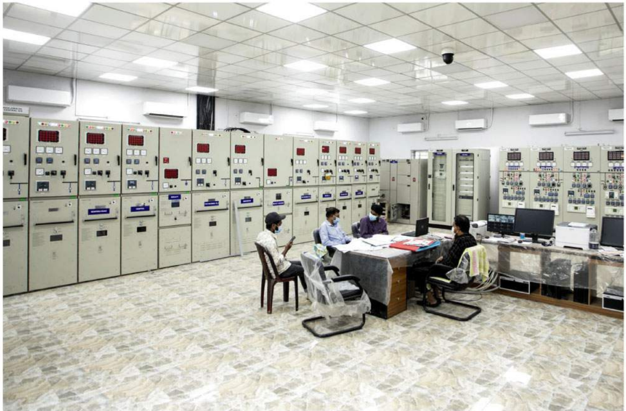
Control Room of Ghope Central 33/11 kV, 2x10/13.33 MVA Substation at Jashore
