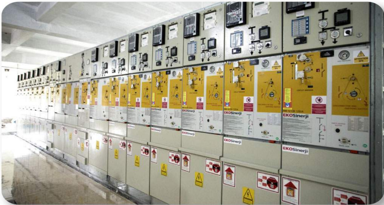
Control Room of Newly Constructed GIS Substation at Moheshorpasa, Khulna
