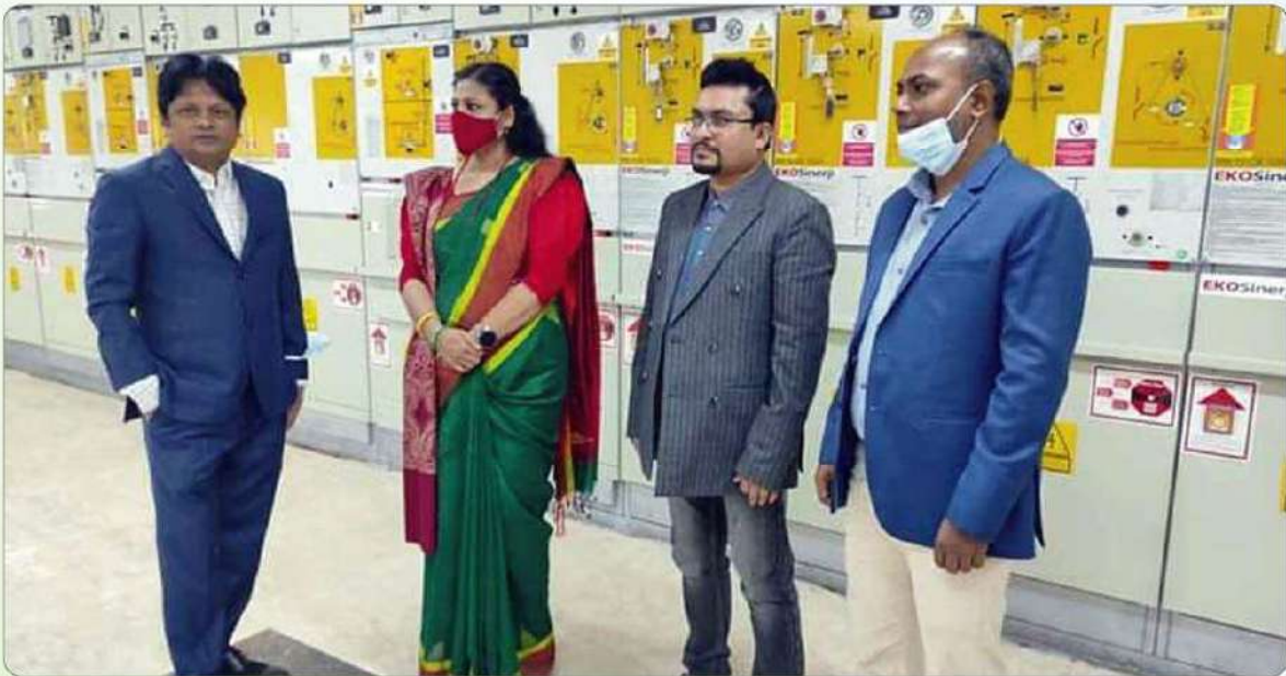
Maksuda Khandaker, Deputy Secretary, Power Division visiting newly constructed sub-station at Khulna
