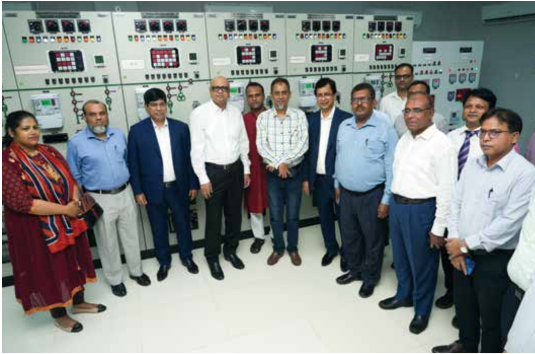
Visit to the newly constructed 33/11 kV Sub-Station at Fultala, Khulna by the Ex-Chairman of WZPDCL Mr. Md. Nurul Alam (Secretary, Energy & Mineral Resources Division)
