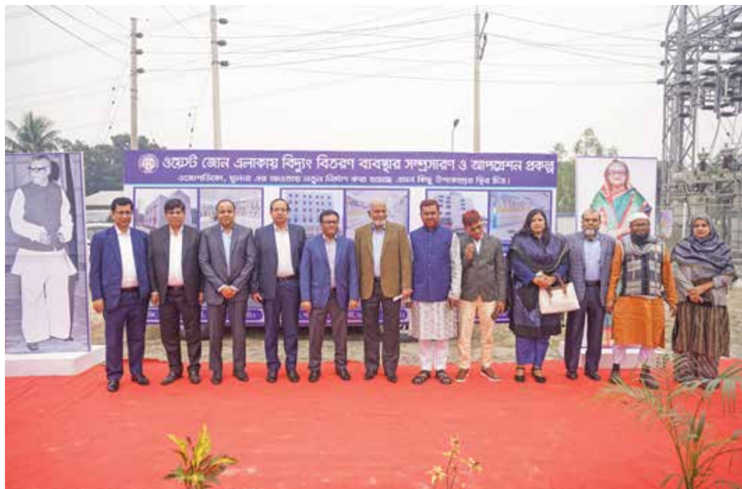
Inauguration ceremony of the newly constructed 33/11 kV Sub-Station at Kaburhat, Kushtia by the Senior Secretary of Power Division Mr. Md. Habibur Rahman, BPAA
