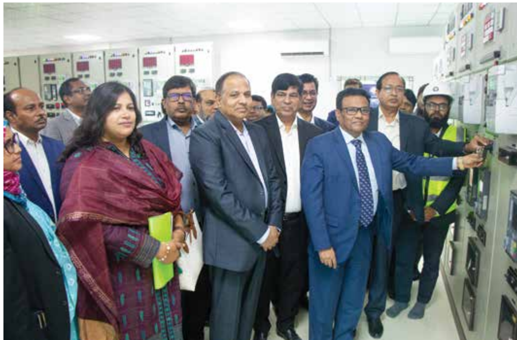
Inauguration ceremony of the newly constructed 33/11 kV Sub-Station at BSCIC, Jashore by the Senior Secretary of Power Division Mr. Md. Habibur Rahman, BPAA
