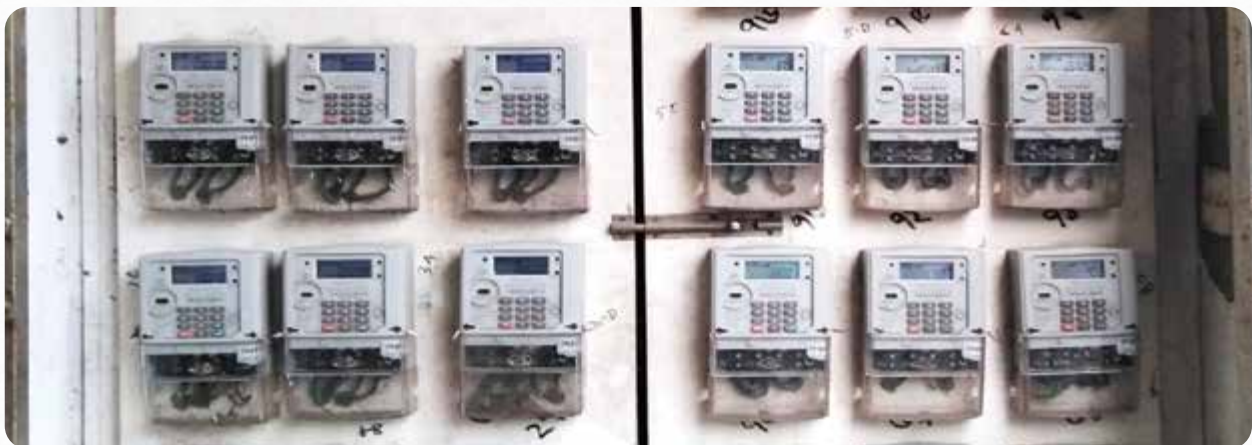
Installed Pre-payment Meter under "Smart Prepayment Metering Project for West Zone Power Distribution Company Ltd. (WZPDCL) Area" project.
