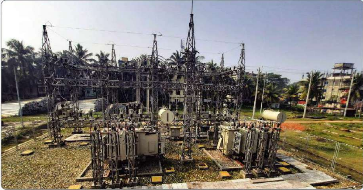
Newly constructed Chanmari, Barishal 33/11kV, 2*10/13.33 MVA Substation
