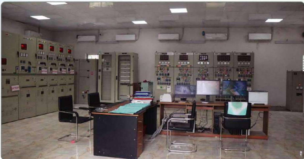
Control Room of Newly constructed Binodpur, Rajbari 33/11kV, 2*10/13.33 MVA Substation
