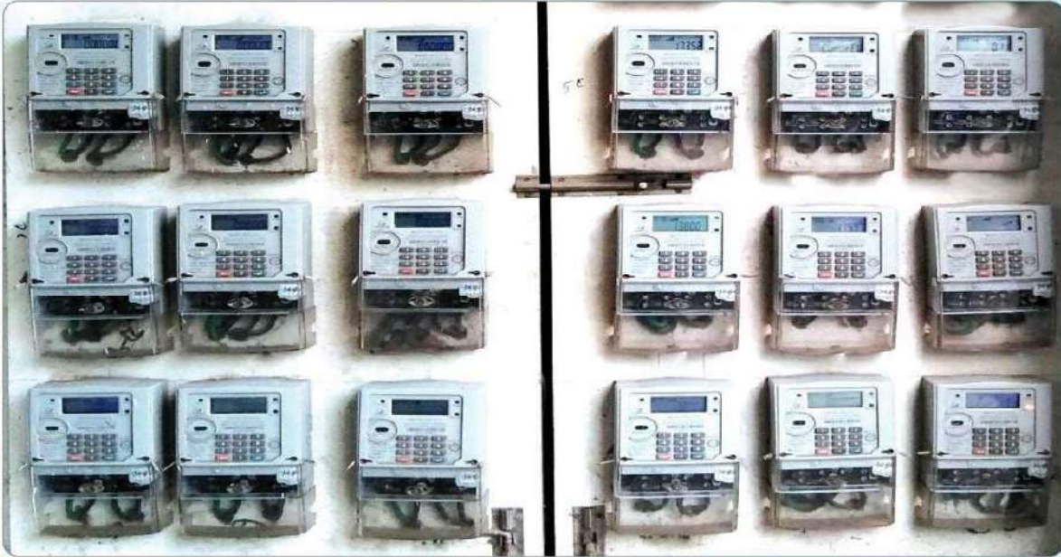
Pre-Payment Meter Installed under Smart Pre-Payment Metering Project.
