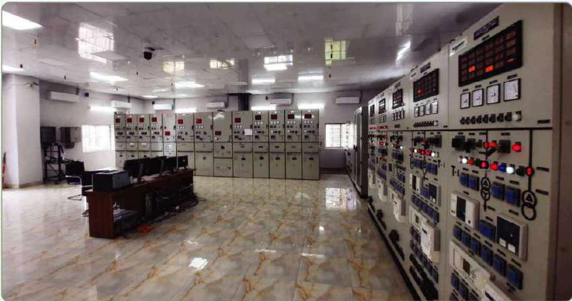
Control Room of Newly constructed Chanmari, Barishal 33/11kV, 2*10/13.33 MVA Substation
