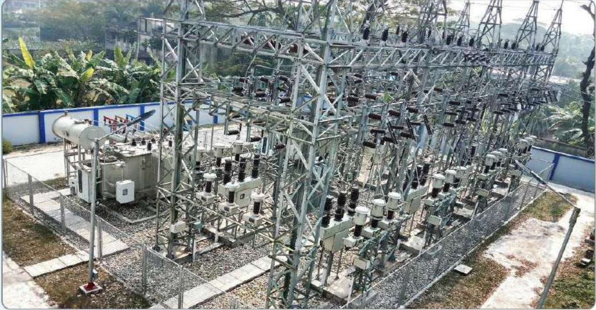
Newly constructed Charfashion 33/11kV, 2*10/13.33 MVA Substation
