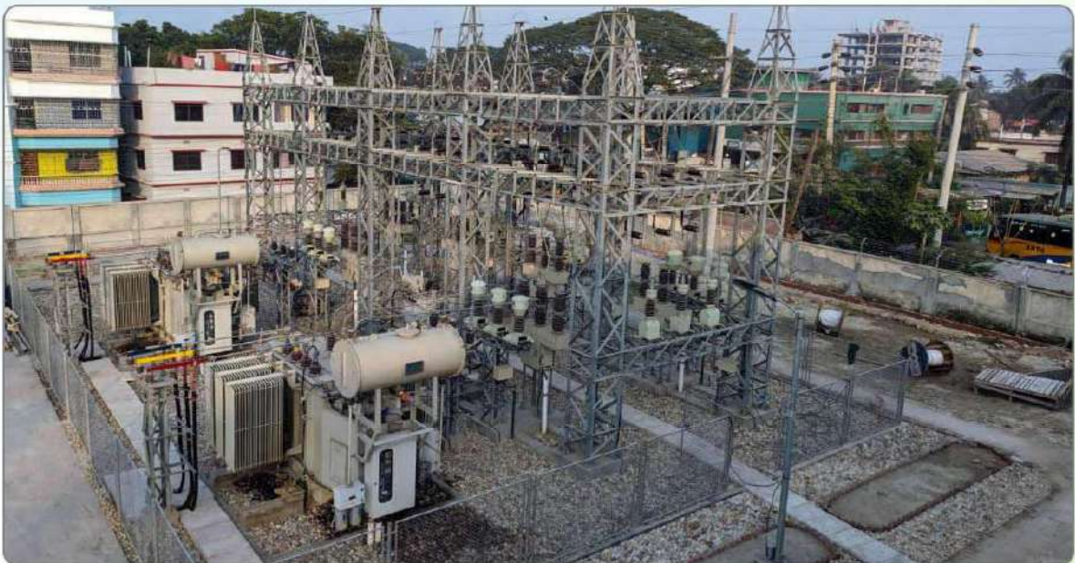
Newly constructed Jhinaidah Campus 33/11kV, 2*10/13.33 MVA Substation
