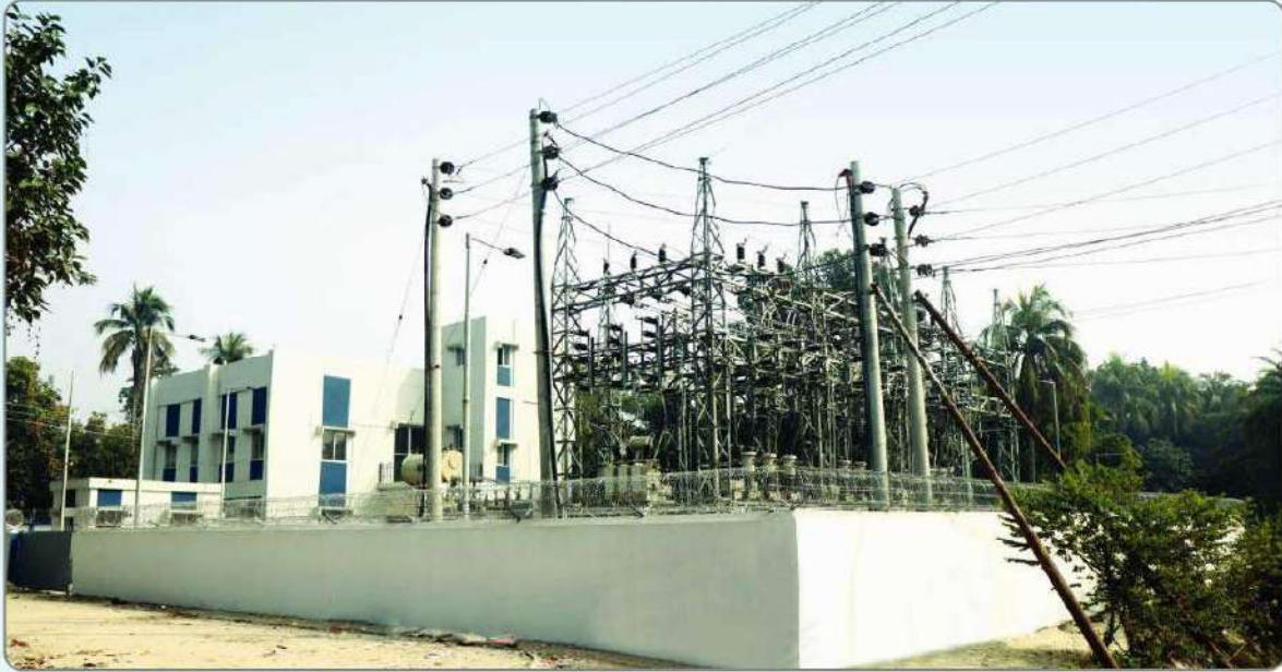
Newly constructed Binodpur, Rajbari 33/11kV, 2*10/13.33 MVA Substation
