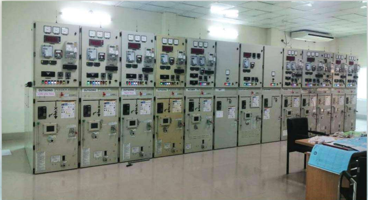
Newly Constructed 33/11 KV Sub-Station Control Room, Jhinaidah.
