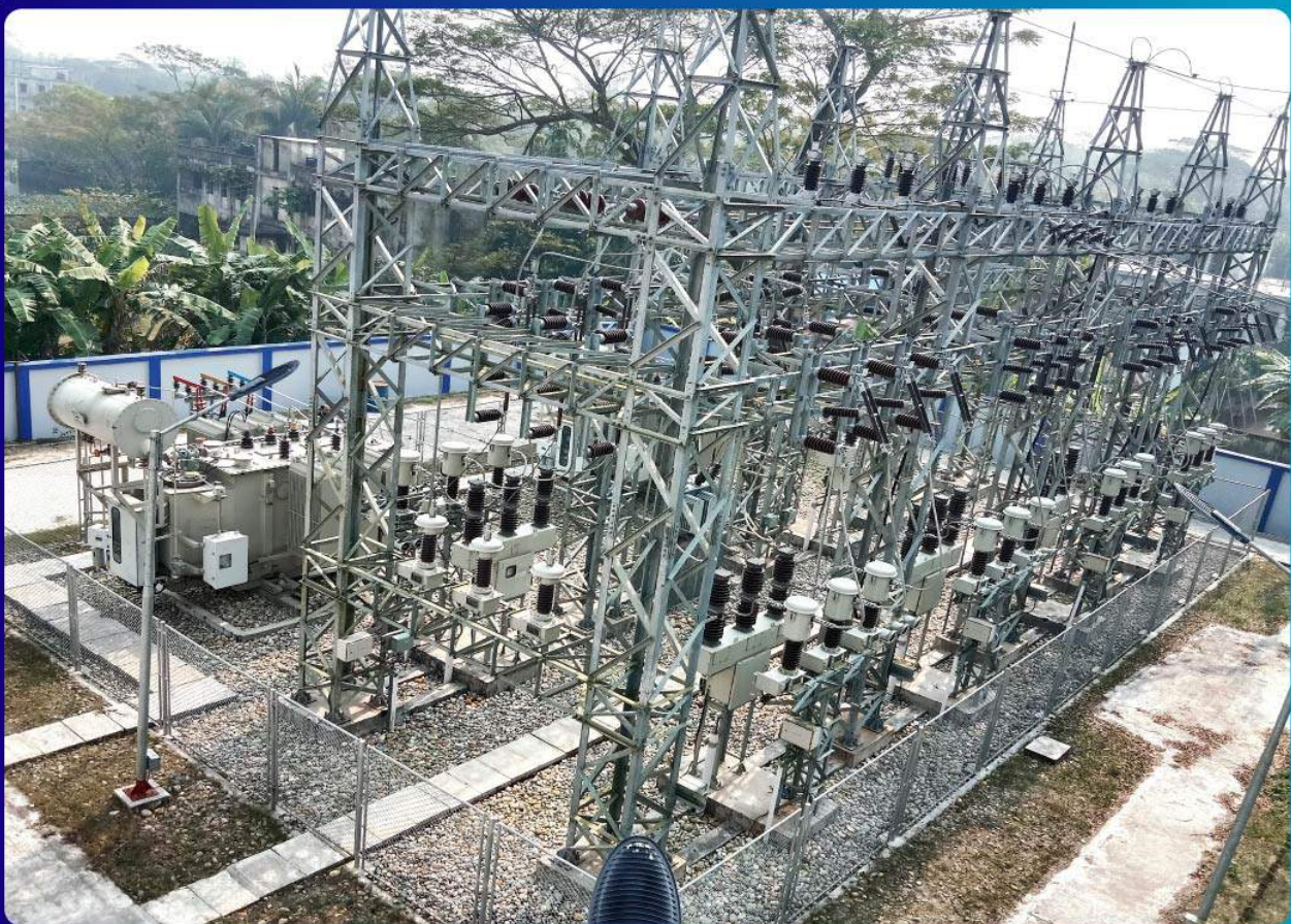
Newly constructed Charfashion 2*10/13.33 MVA, 33/11kV Sub-Station.
