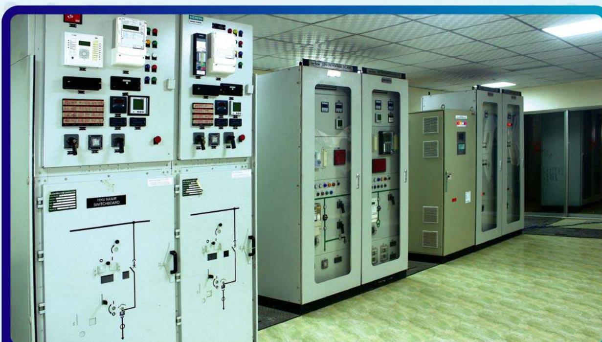
Control Room, Model Sub-Station, WZPD Training Institute, Khulna.
